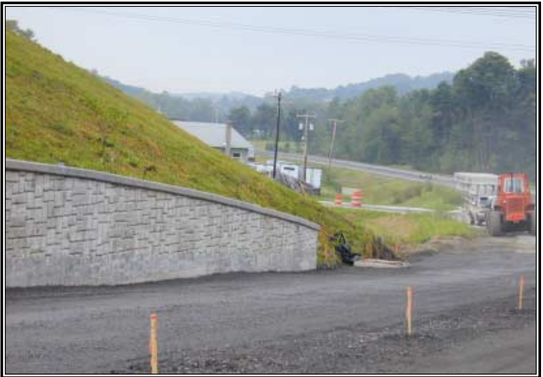
Retaining walls on project storage sites, drainage and major earthwork can be seen in the mountains of Western Maryland
