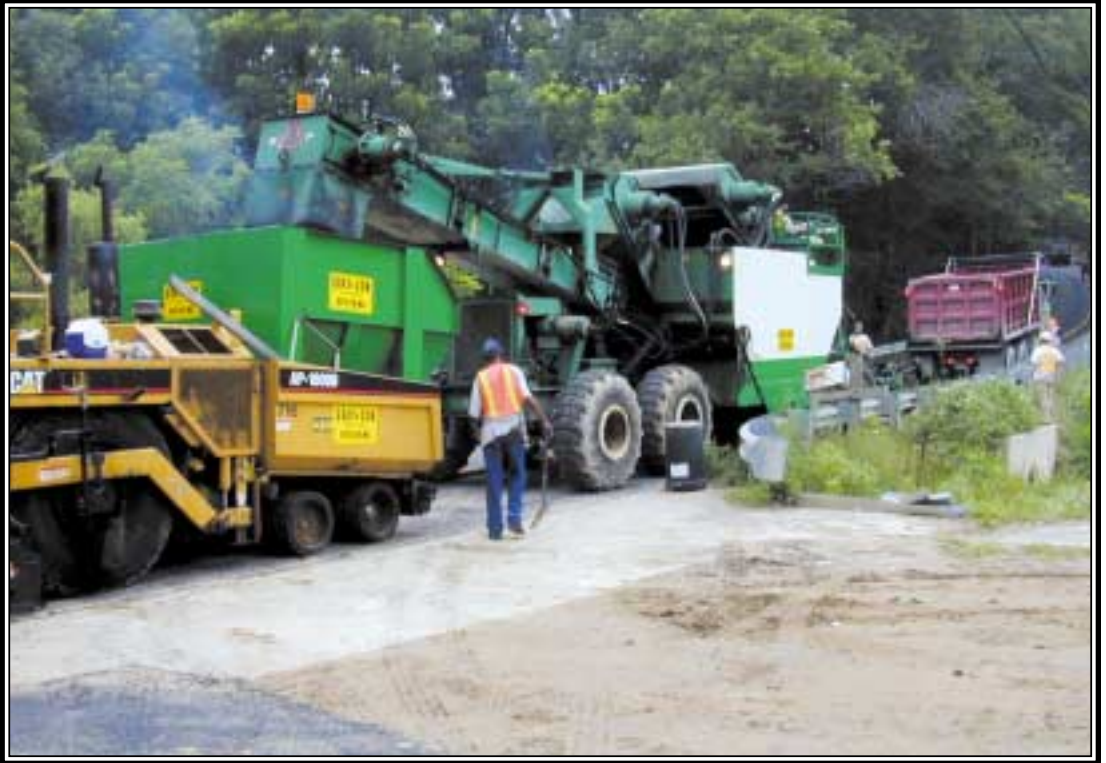
Older Barber Greene material transfer device feed HMA to the hopper of a new rubber tired CAT paver. This process improves ride and eliminates segregation.
