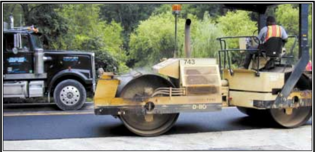
Large Ingersoll-Rand D-110 rollers are used to achieve density on this project.
