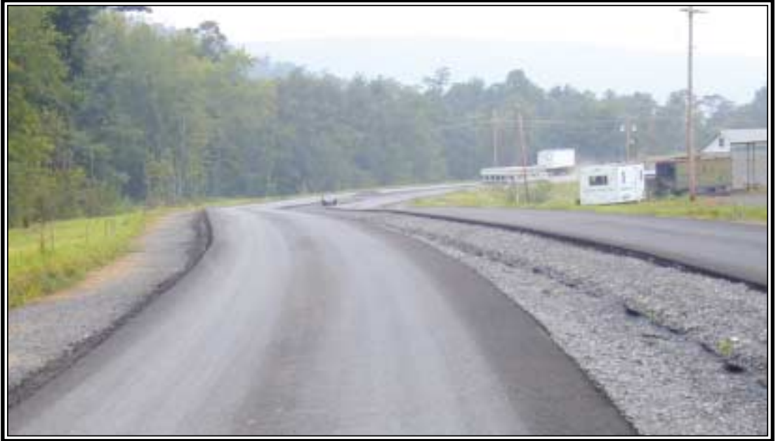
19 MM Superpave Base course is in place on the West Virginia end of the project.
