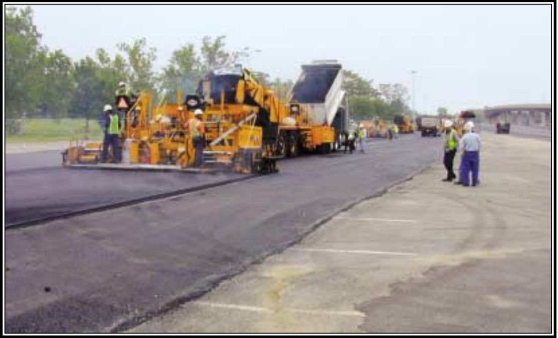
Fully extended screeds were fed by material transfer devices and a steady stream of trucks.
