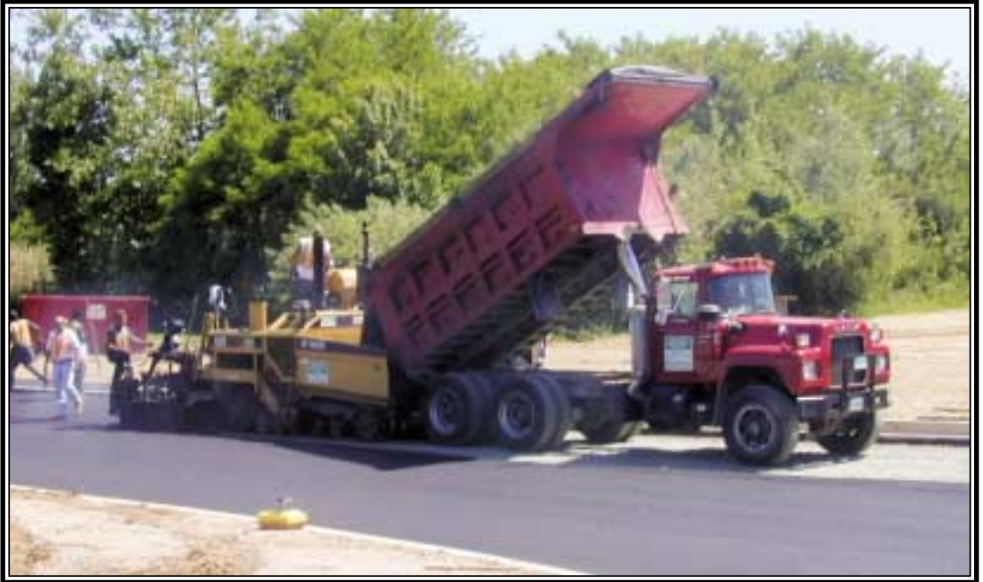
Entrance reconstruction operation demonstrated paving within confined areas. Densities were verified by Troxler Nuclear Density Gauge.
