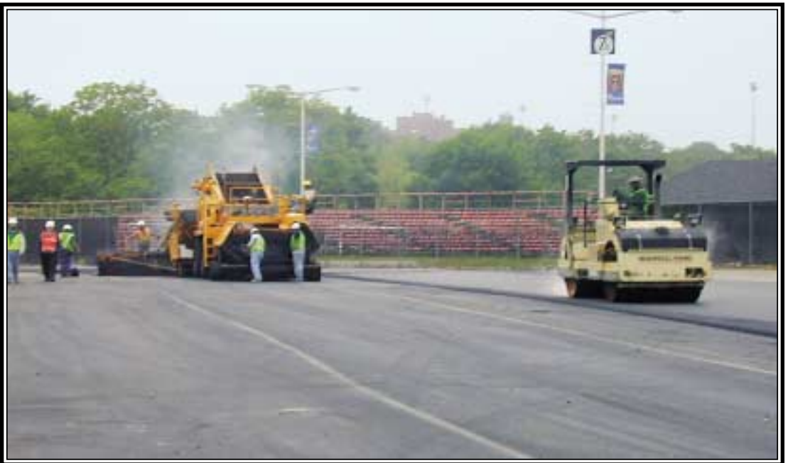
The second paver exits a tight corner while the intermediate roller compacts mix in next lane.
