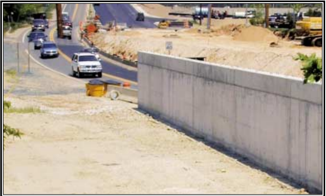
New retaining wall at Lowes helps accomplish significant grade change while staying within the existing right of way.
