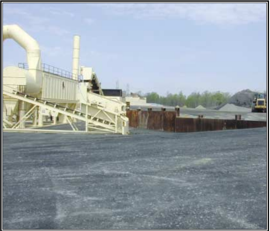
Retaining wall at the cold feed system is constructed from salvage materials originally incorporated in the Georgetown Trolley Line.
