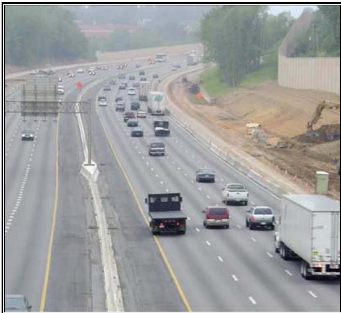
Cherry Hill Contractors widen I-95 and install noise walls prior to final SMA lift by P. Flanigan & Sons, Inc..
